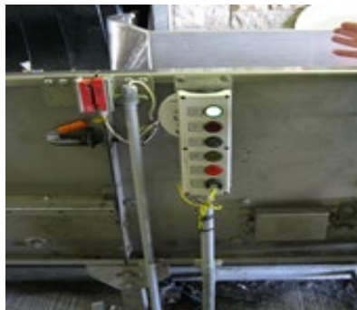
REMOTE (EXTERNAL) OPERATOR CONTROL STATION
