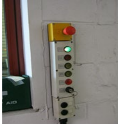
REMOTE (INTERNAL) OPERATOR CONTROL STATION
